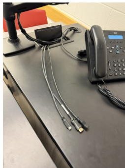
Cable access at the tabletop
